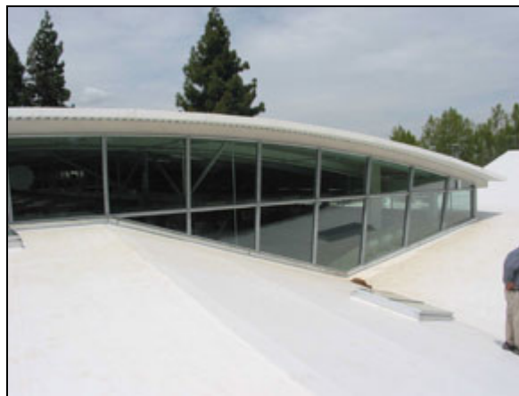
Figure 6.2: Example of a cool roof (fypower.org).
